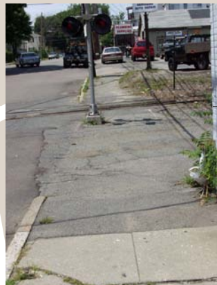
Disrepair near railroad tracks
