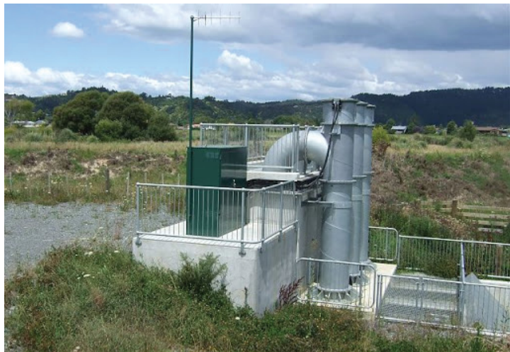
Stormwater pump station
