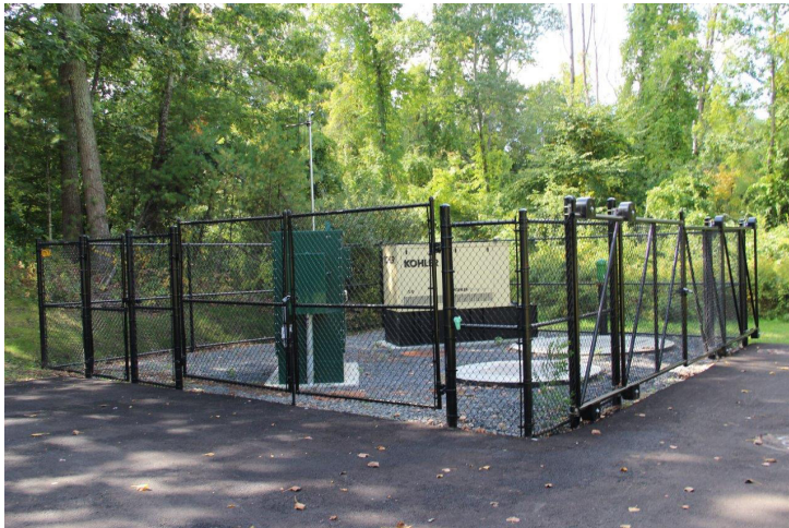
Sewer pump station
