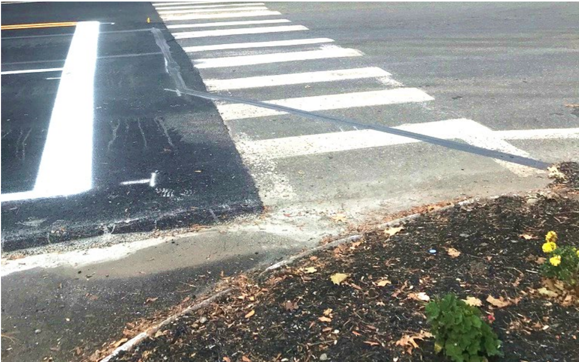
Figure 14 Lack of Pedestrian Facilities on Southwest Intersection Corner leading to Great Road (Route 117) Crosswalk
