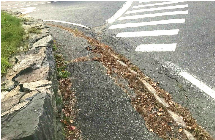
Figure 16 Southeast Intersection Corner Crosswalk Lacking Pedestrian Facilities
